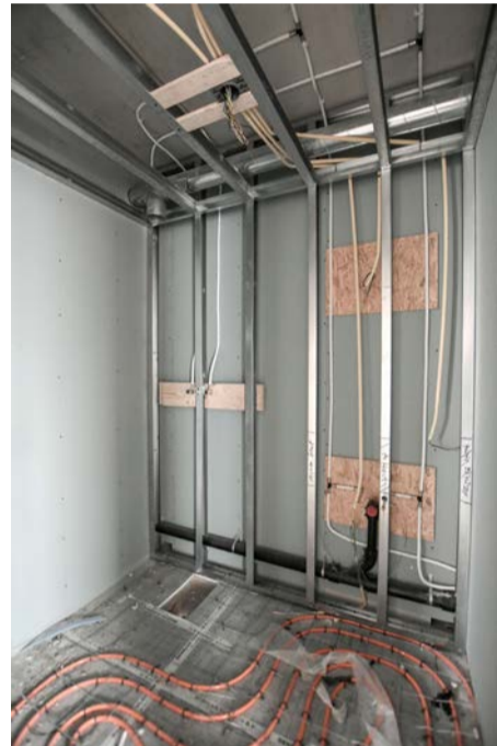
The adaptable installations behind a suspended ceiling and false facing wall
