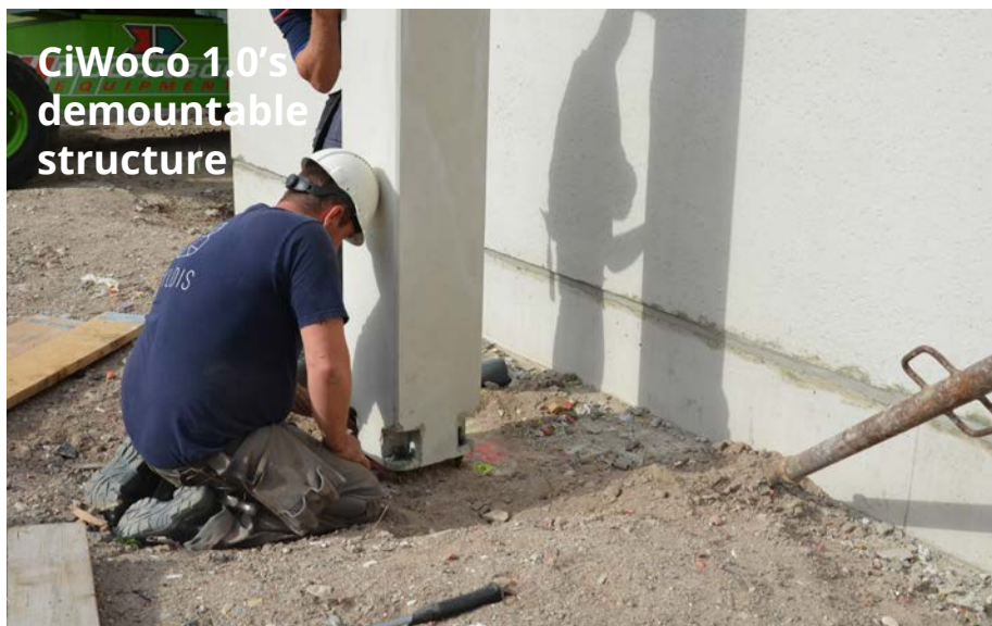
Together with the contractor, structural engineer and concrete suppliers, Bestcon and Peikko, demountable connections were developed for the prefab concrete shell
